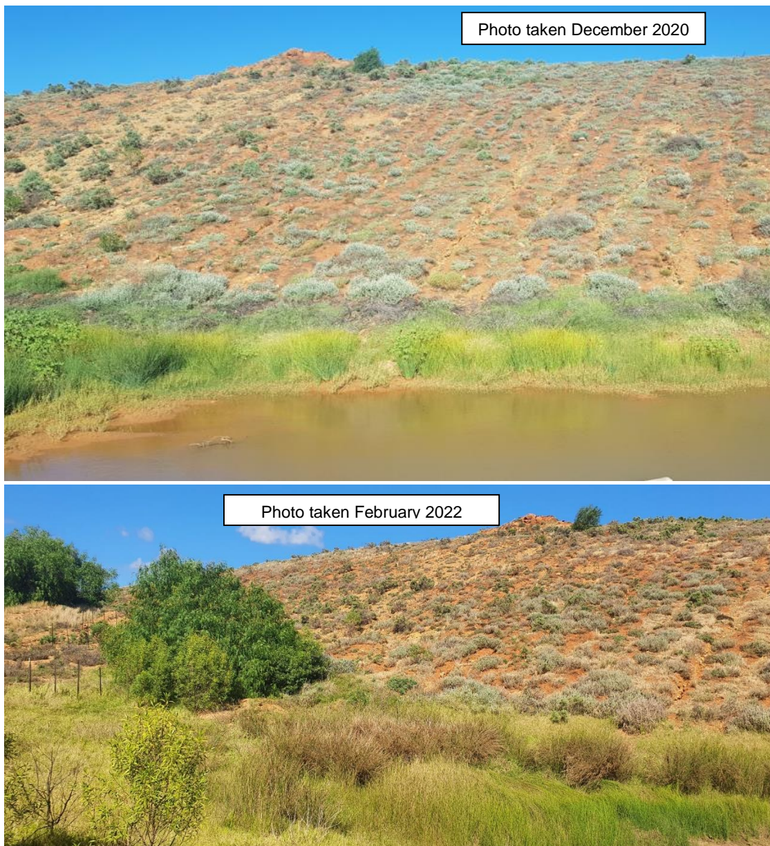
Figure 3: Comparative photos of the Eastern bank of the waste rock emplacement showing progress of groundcover species growth and minimal erosion.
