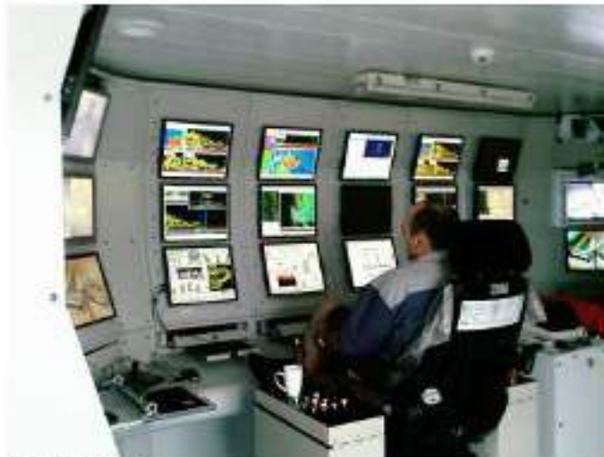
Figure 4-10: Typical operator control console.
