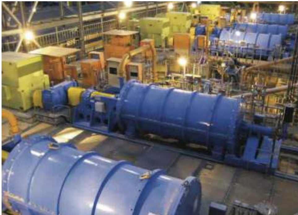
Figure 7-22 M10,000 IsaMills™. Installation, South Africa
